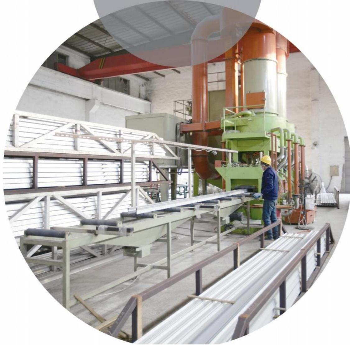
喷砂机 Sandy blasting equipment
